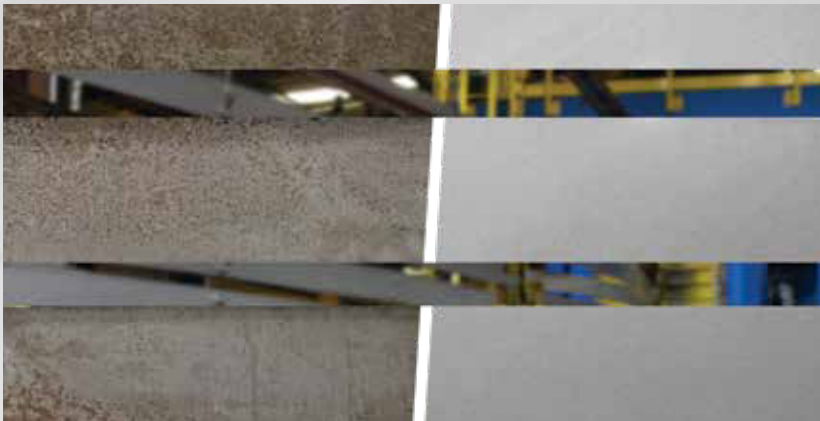
After blasting, the steel is in near white metal condition in compliance with SSPC 10/ NANCE and SSPC 5.1.4. standards.
