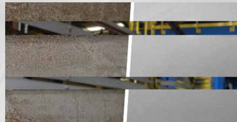
After blasting, the steel is in near white metal condition in compliance with SSPC 10/ NACE and SSPC 5.1.4. standards.
