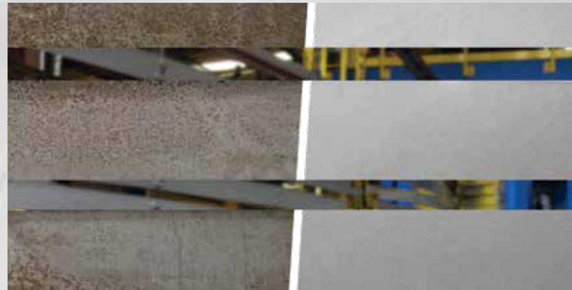
After blasting, the steel is in near white metal condition in compliance with SSPC 10/ NACE and SSPC 5.1.4. standards.
